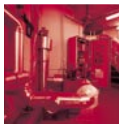
■ Air conditioning units
